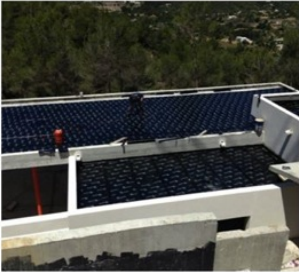
Roof top with solar panels
